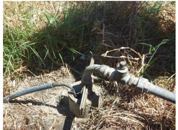
Original Borehole & Pump (now decommissioned)
