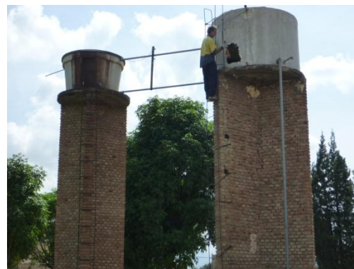
Fibre-glass elevated tank in disrepair
