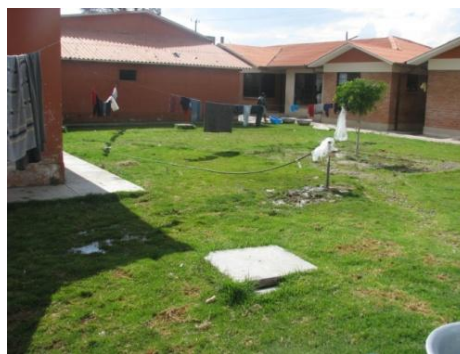
Taps broken wasting water
