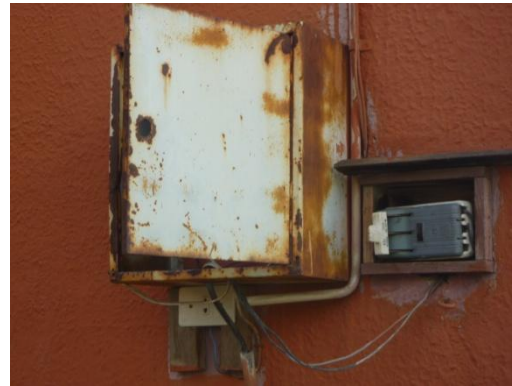
Unsafe pump electrical connection
