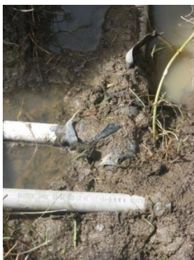
Pipe systems broken & leaking
