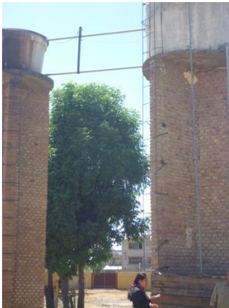
2 x Elevated Water Tanks on 6mtr High Stands
