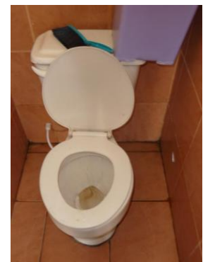
Toilet cisterns damaged wasting water
